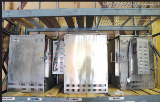
View of Paragon Furnaces
