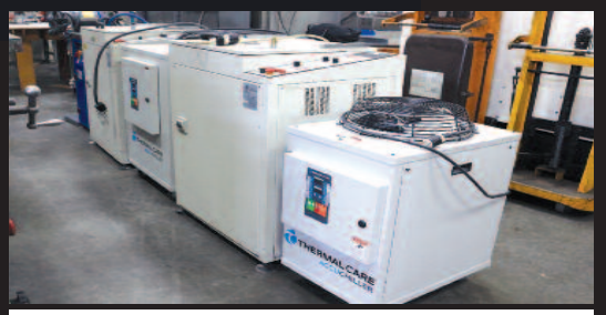
View of Furnaces and Chillers
