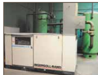
(1 OF 2) 1996 INGERSOLL-RAND 100 HP ROTARY SCREW AIR COMPRESSORS
