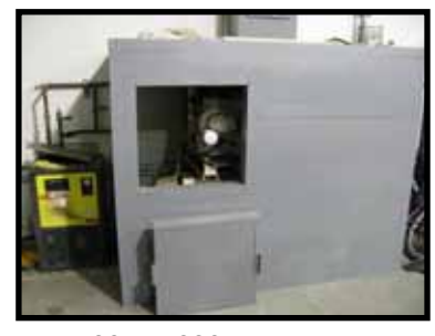
IR AIR COMPRESSOR W/ ZEK'S DRYER
