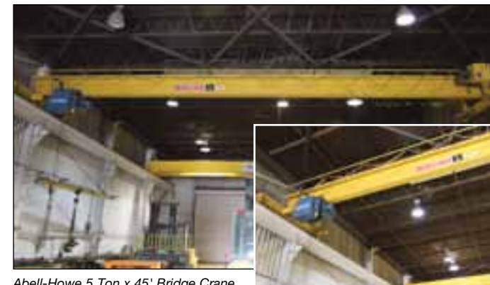
Abell-Howe 5 Ton x 45' Bridge Crane
